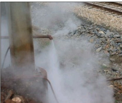
FIGURE 4. Visual inspection shows that there is clearly liquid being discharged with the steam, indicating poor quality
