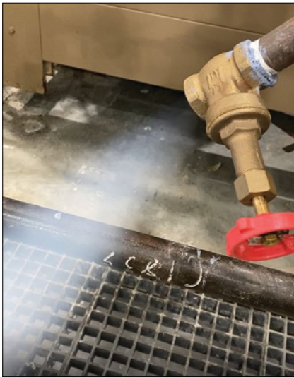
FIGURE 2. Visual inspection can be used to show that steam is of acceptable quality. The steam should be nearly invisible
